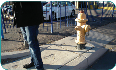
A fire hydrant blocks the sidewalk along Central at Cardenas.
