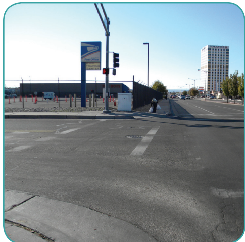
A crosswalk at Central and Alvarado with faded and missing paint.
